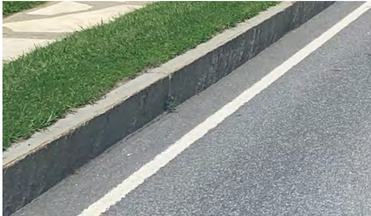
The sharp granite curbs and narrow shoulders are dangerous for cyclists.
